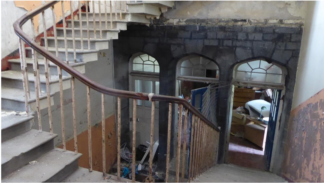
Figure 11 Secondary Staircase as seen from half landing looking down to ground floor level of service range © Holland Heritage
